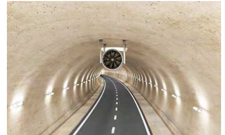
Ventilatori in tunnel.
